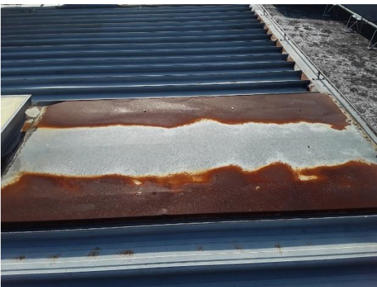
Rust damage that could cause future problems.
