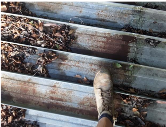
The damaged sealant causing the roof leak.
